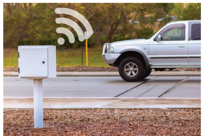
The roadside cabinet includes a solar panel, back up battery & modem that securely transmits data remotely.
