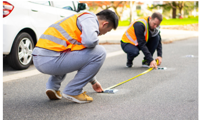
Installation is quick and easy. Taking the time to position the magnetometers in a precise array ensures optimum data quality.
